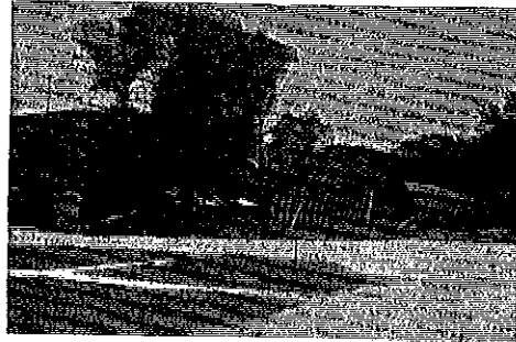
VIEW of the new Fire Hall being constructed presently. Familiar City Hall is at left.
